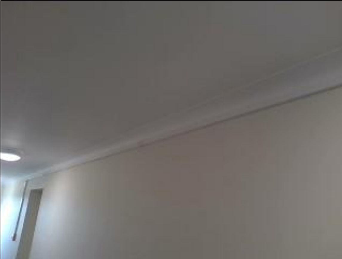
25812_Action_Consider replacing plastic cable c_15
