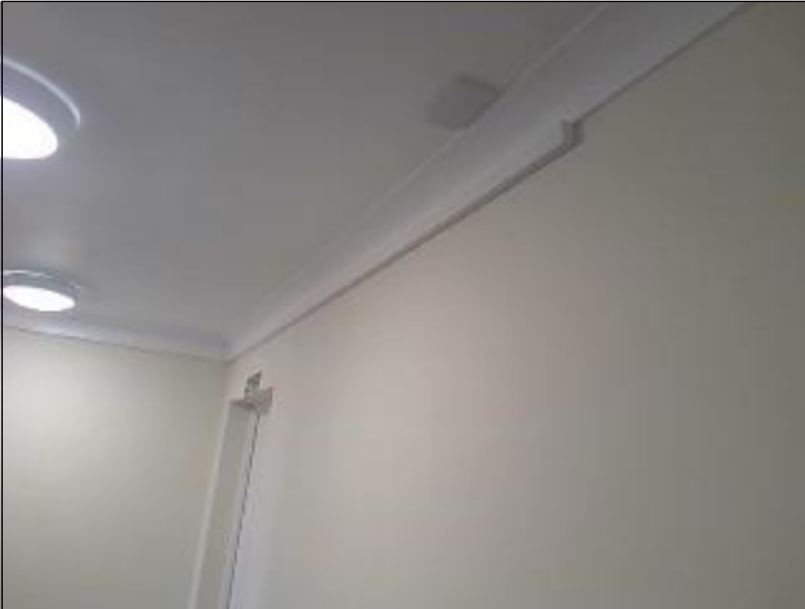
25812_Action_Consider replacing plastic cable c_08
