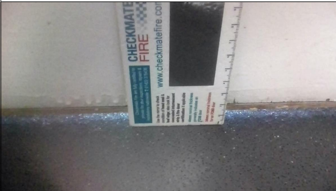
23030_Action_The following doors require mainte_06
