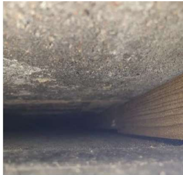
Photo 4: Adjacent to window reveal showing clear cavity and timber battens behind Trespa Meteor panel.
