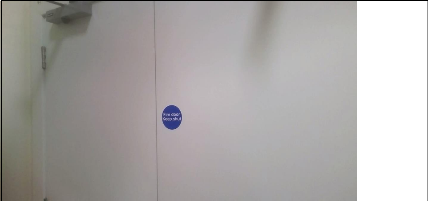
22324_Action_Another action or repair was ident_04
