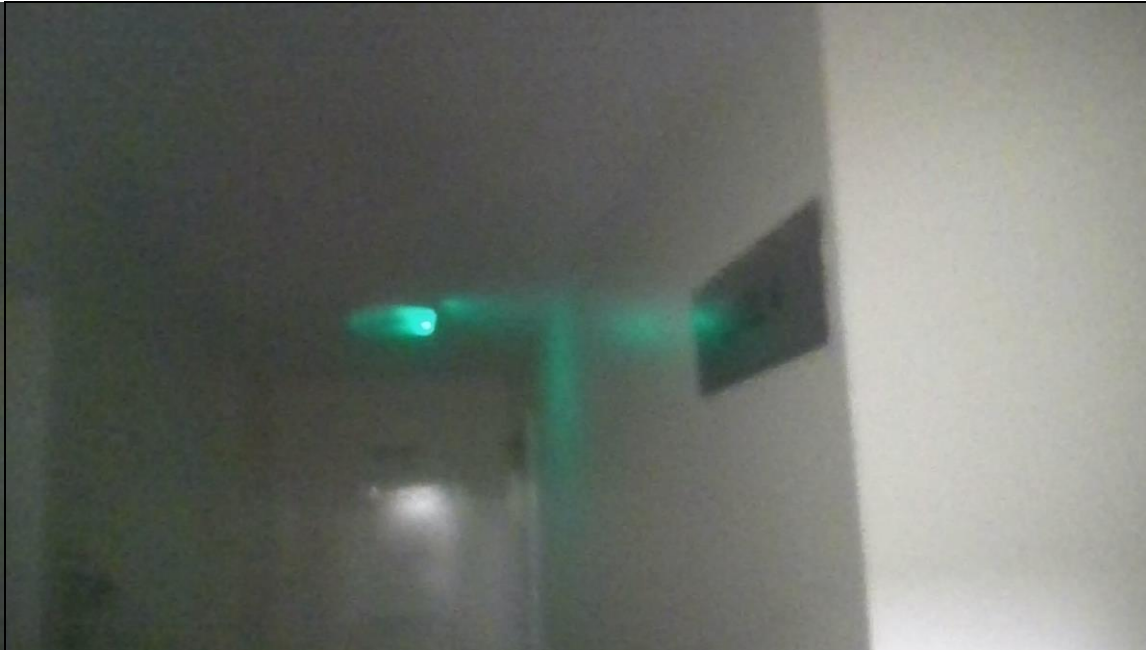
22324_Action_Artificial lighting is damaged and_19
