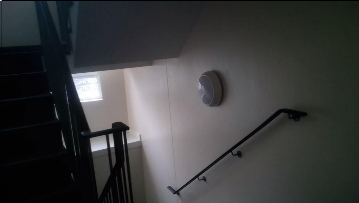
22324_Action_Artificial lighting is damaged and_06
