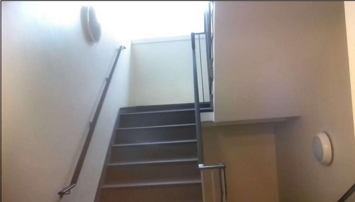
22324_Action_Artificial lighting is damaged and_08
