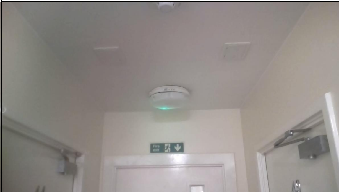
22324_Action_Artificial lighting is damaged and_07
