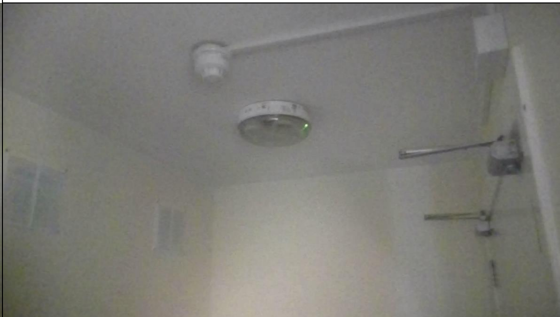
22324_Action_Artificial lighting is damaged and_12
