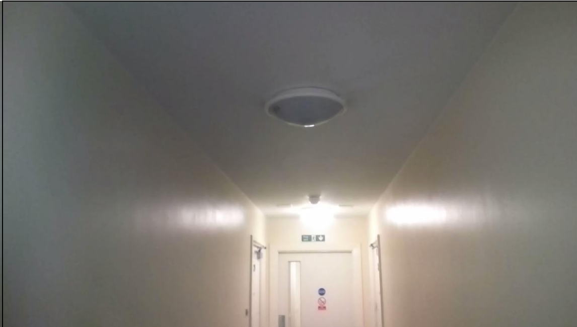
22324_Action_Artificial lighting is damaged and_11
