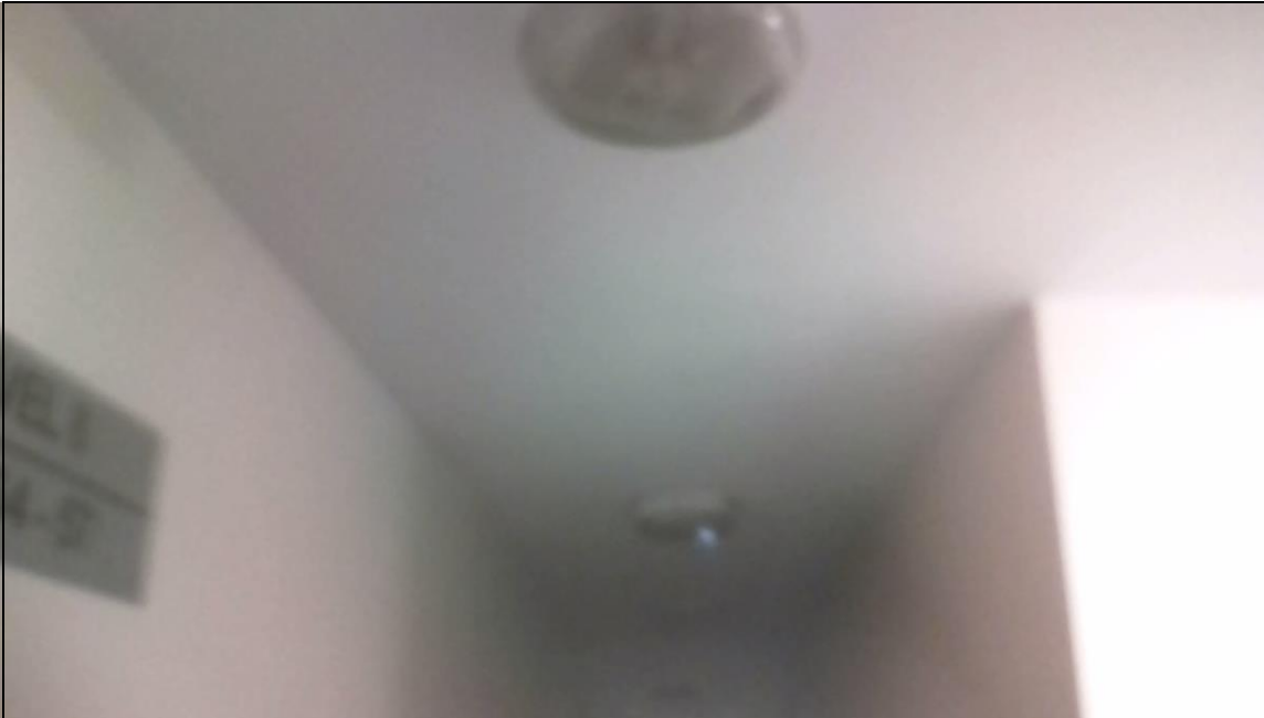
22324_Action_Artificial lighting is damaged and_03
